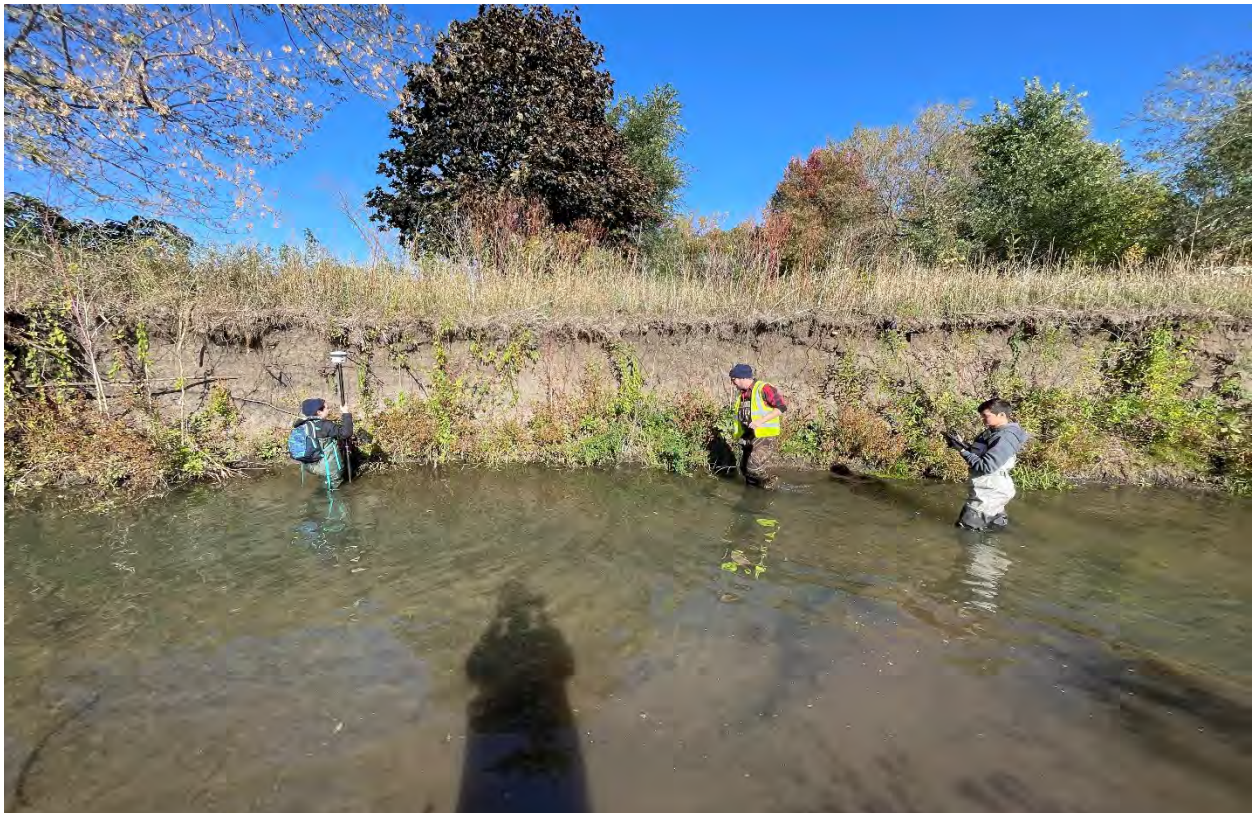
Photo point 21: Bear Creek looking southwest. Severely eroded bank shows degree of stream incision. Date taken: October 10, 2023
